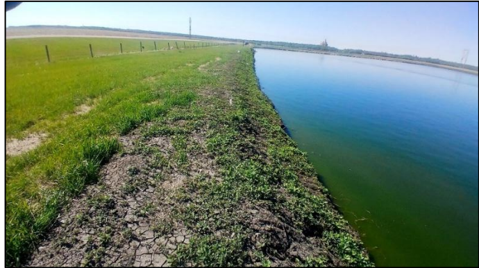
Figure 3 Erosion along the eastern shoreline of Cell 2
